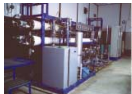
Field test system in Okinawa
