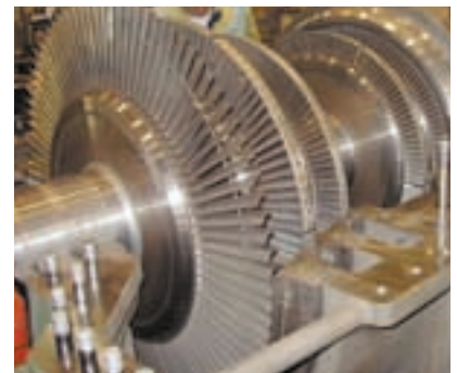
Steam turbine that produces electricity
