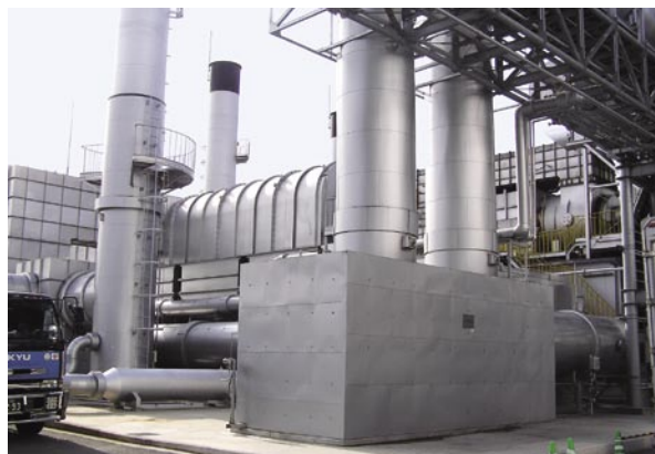
Deodorizing furnace in the Onomichi Plant
