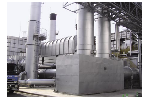
Deodorizing furnace in the Onomichi Plant
