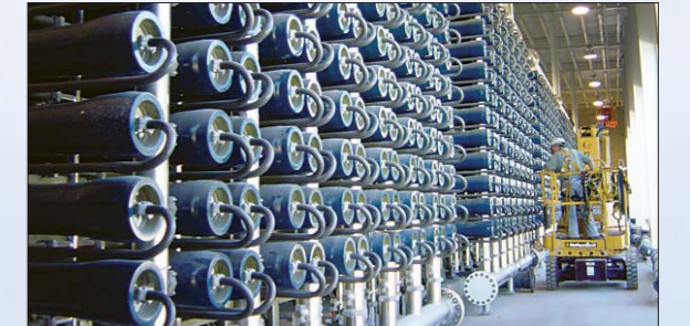
Reserve osmosis membrane for seawater desalination
