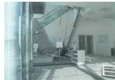
Damage to the Nitto Denko Tohoku Plant Part of the ceiling above the stairs in the building collapsed.
