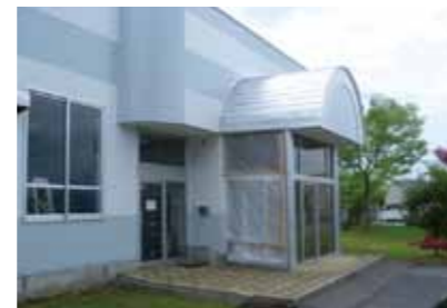
Nissho Iwaki Plant The glass in the entrance was broken. (Part covered with film)
