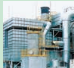
■ Deodorizing furnace (with waste heat boiler)
