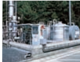
■ RO unit for recovering solvents
