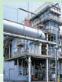
■ Solvent recovery unit
