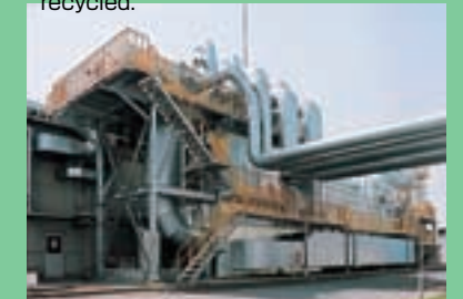
■ Deodorizing furnace installed at Nitto group company Nitto Shinko Corp.
