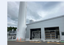
Hydrogen Utilization Facility
