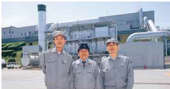
The new deodorizing furnace
