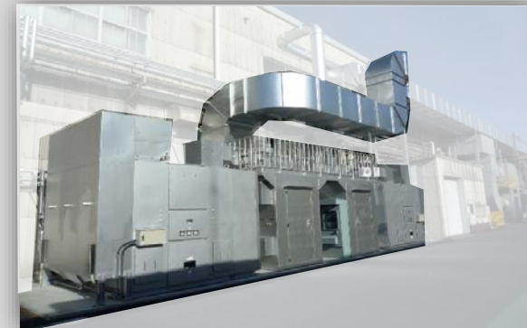
Exhaust Treatment Facility at Toyohashi Plant (Established in FY2017)
