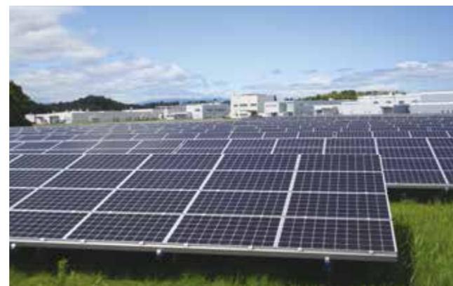
Solar power generation facility at Nitto's Tohoku Plant
