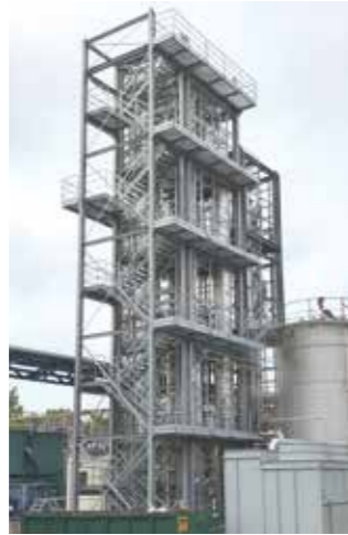
Solvent recycling equipment at Nitto Belgium NV
