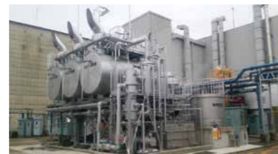
Solvent recovery equipment installed at the Kanto Plant
