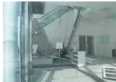
Damage to the Nitto Denko Tohoku Plant Part of the ceiling above the stairs in the building collapsed.
